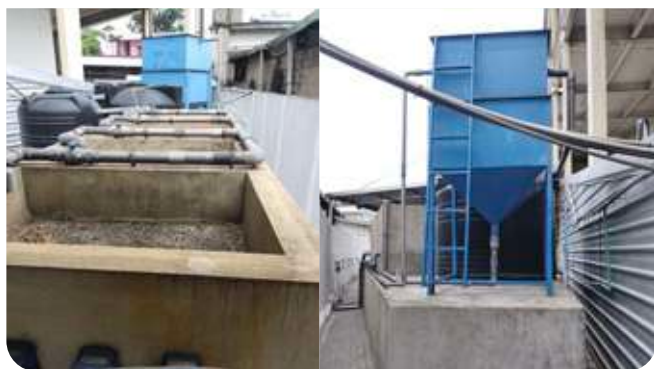
Wastewater treatment plants at JKCG service stations.
