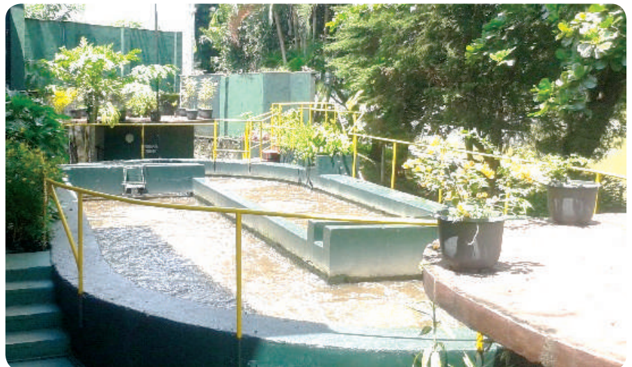
Effluent Treatment Plant at 'Cinnamon Citadel Kandy'.
